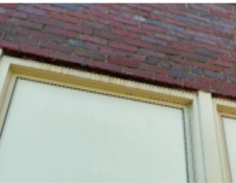
Image 14 – rusting lintels at 1939 wing
