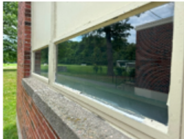
Image 16 – Deteriorated glazing, single pane (1957)
