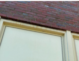
Image 14 – rusting lintels at 1939 wing
